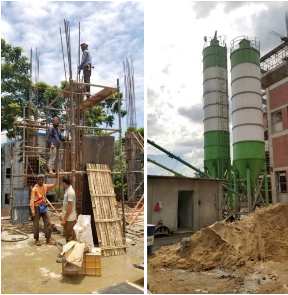
Figure 2: (from left to right) Concrete shuttering, and batching plant. Site: Blueocean footwear factory and Golden Sky footwear factory. Source: Author
