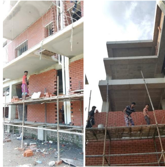
Figure 3: (left to right) Brickwork, scaffolding for brickwork at Golden sky footwear factory. Source: Author
