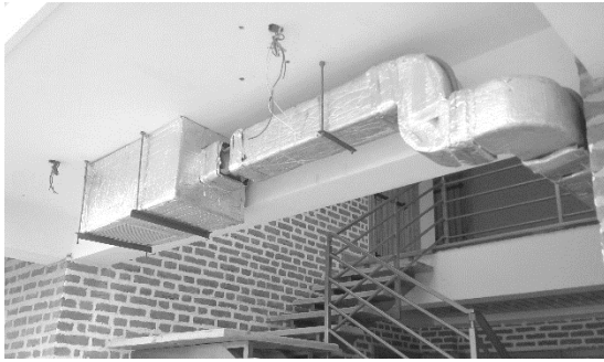
Figure 14: Duct to supply hot air in winter and cold air in summer
