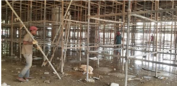
Figure 1: Steel formwork and scaffolding at Blue Ocean Footwear Factory construction site. Source: Author
